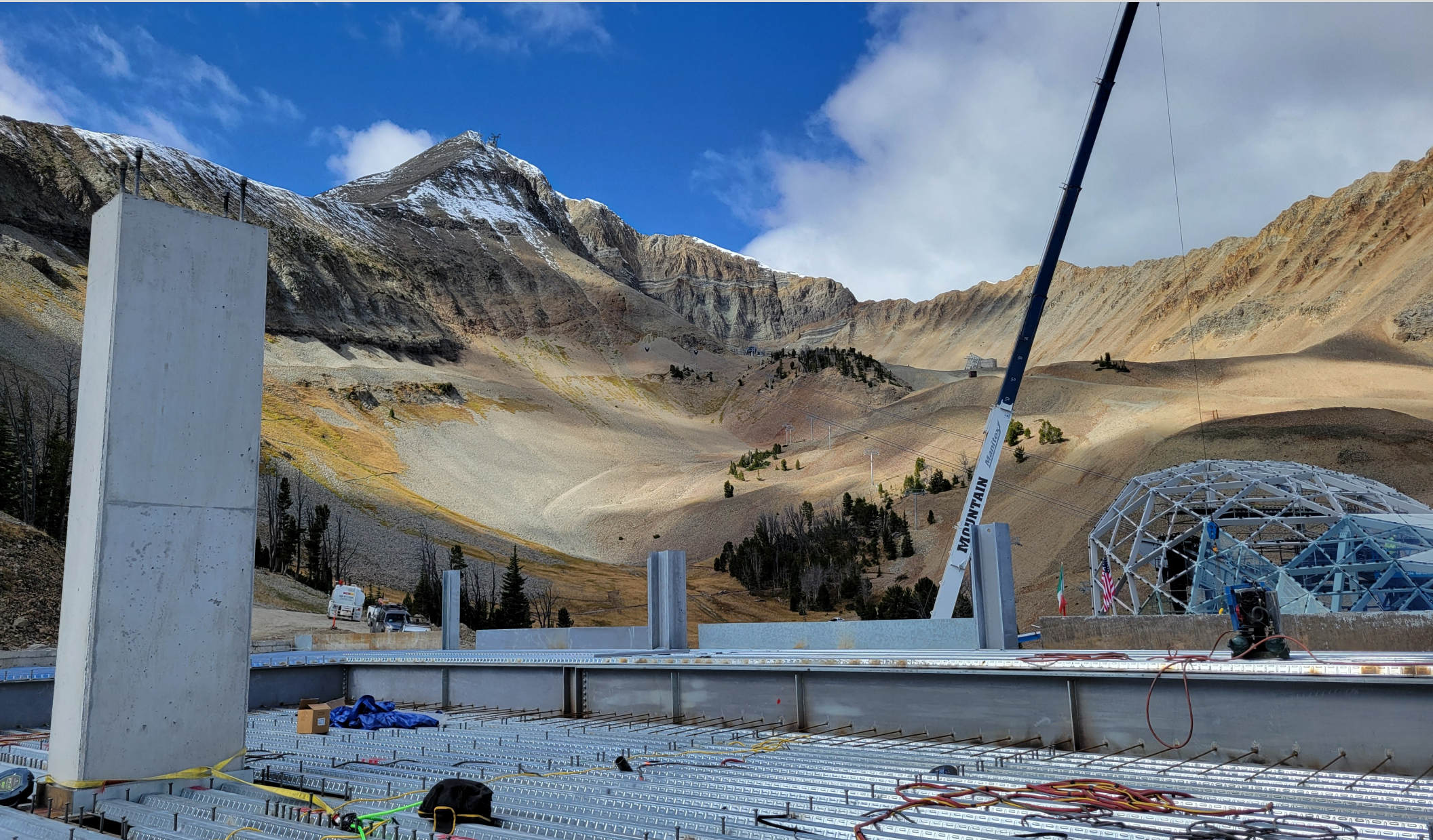
Photo by: Tyson Harvey, Manhattan Plumbing and Heating- Lone Peak, Big Sky Resort's new gondola top-station
